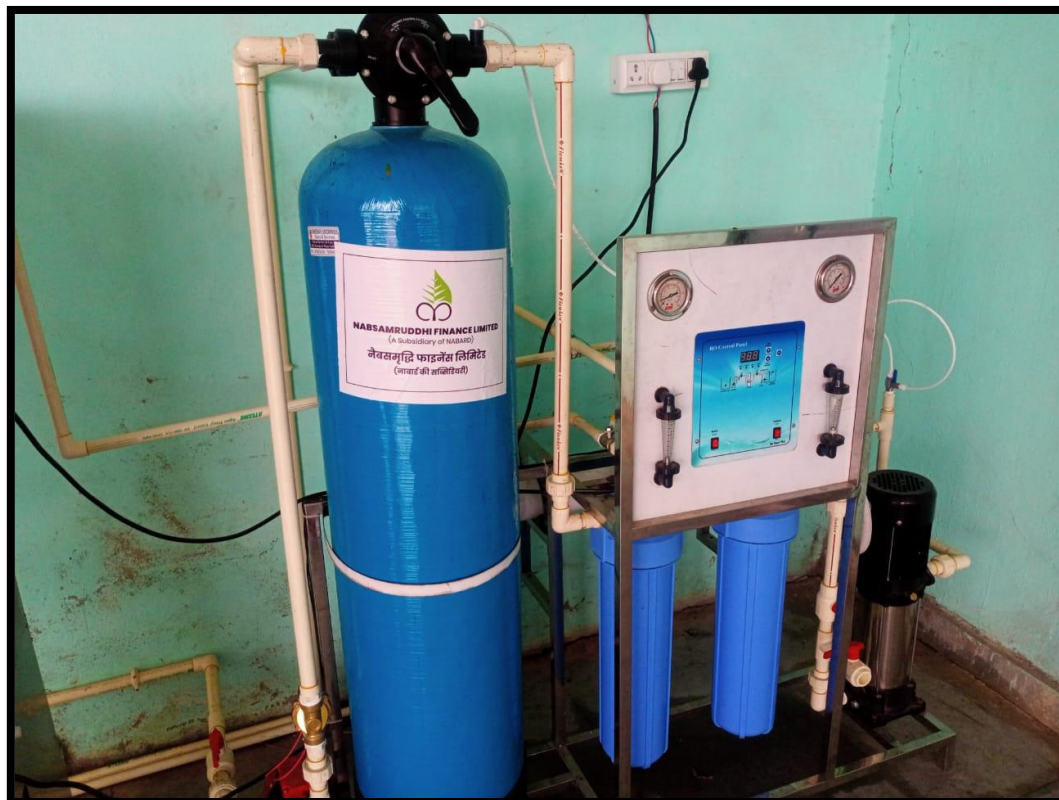
Water Purifier at Education Complex School
